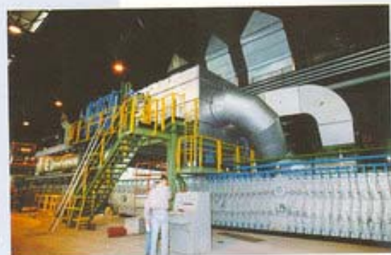
Figure 3. Strip cooling section
