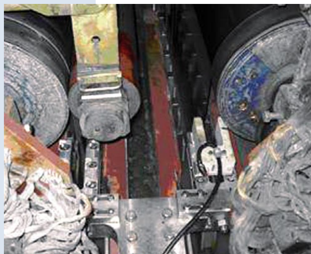
Figure 1. Insoluble anodes are vertically positioned in the plating cell
