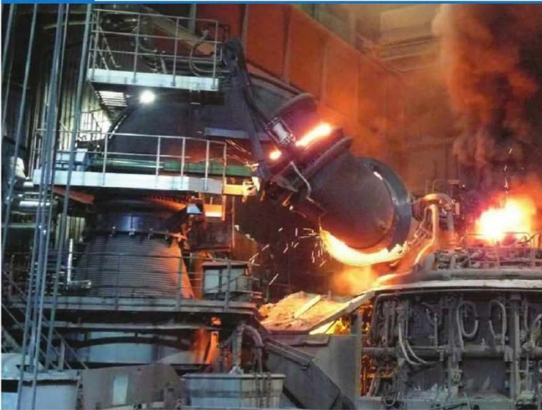
The iRecovery waste gas duct of the EAF in Georgsmarienhütte, Germany.
