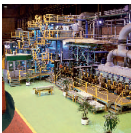
Fig 5 Tin dissolution plant at Ternium Siderar
