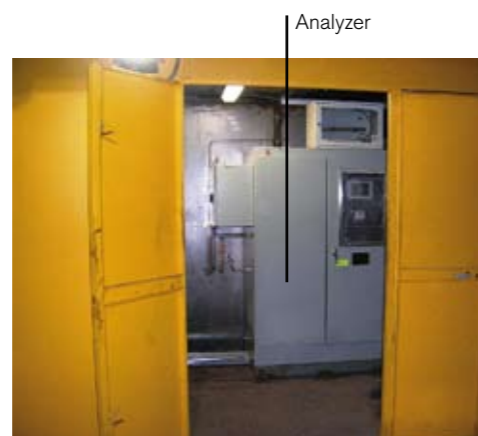
Analyzer room installation.
