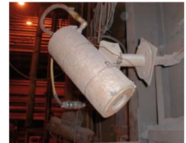
Typical installation of the iBOF® tapping camera.
